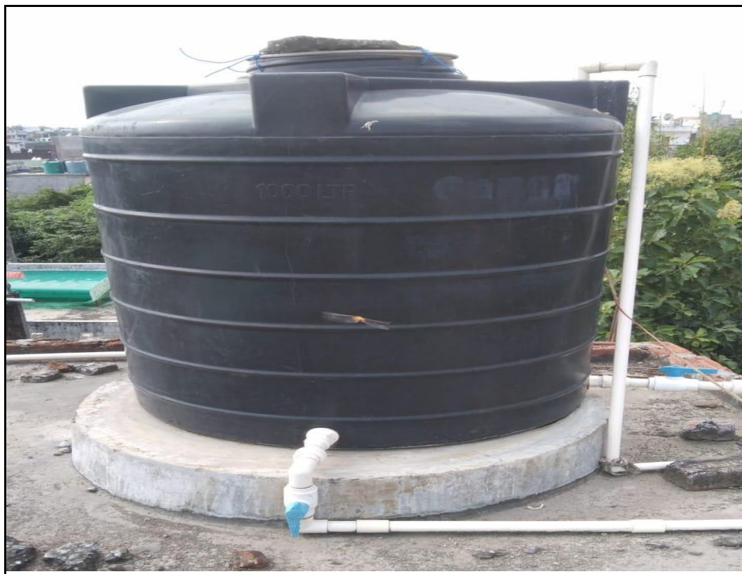
Fig: - 2.2 Water storage tank and capacity of college campus
