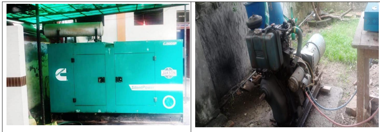
DG set in College Campus
